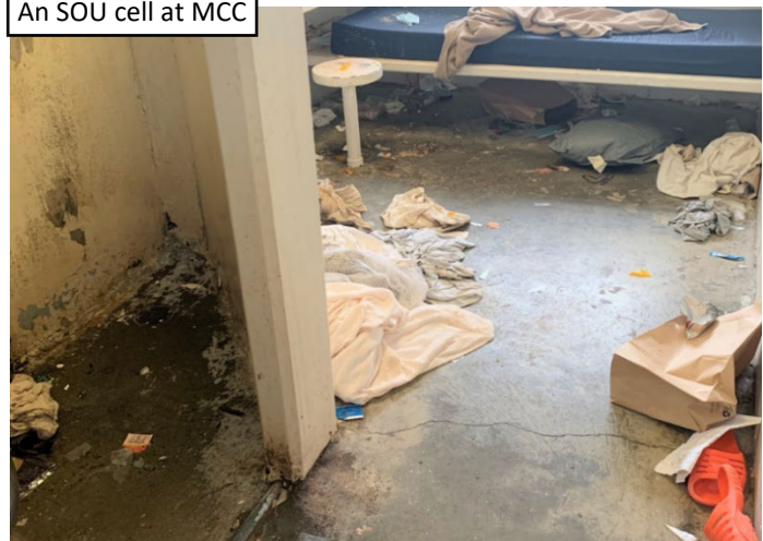
An SOU cell at MCC
